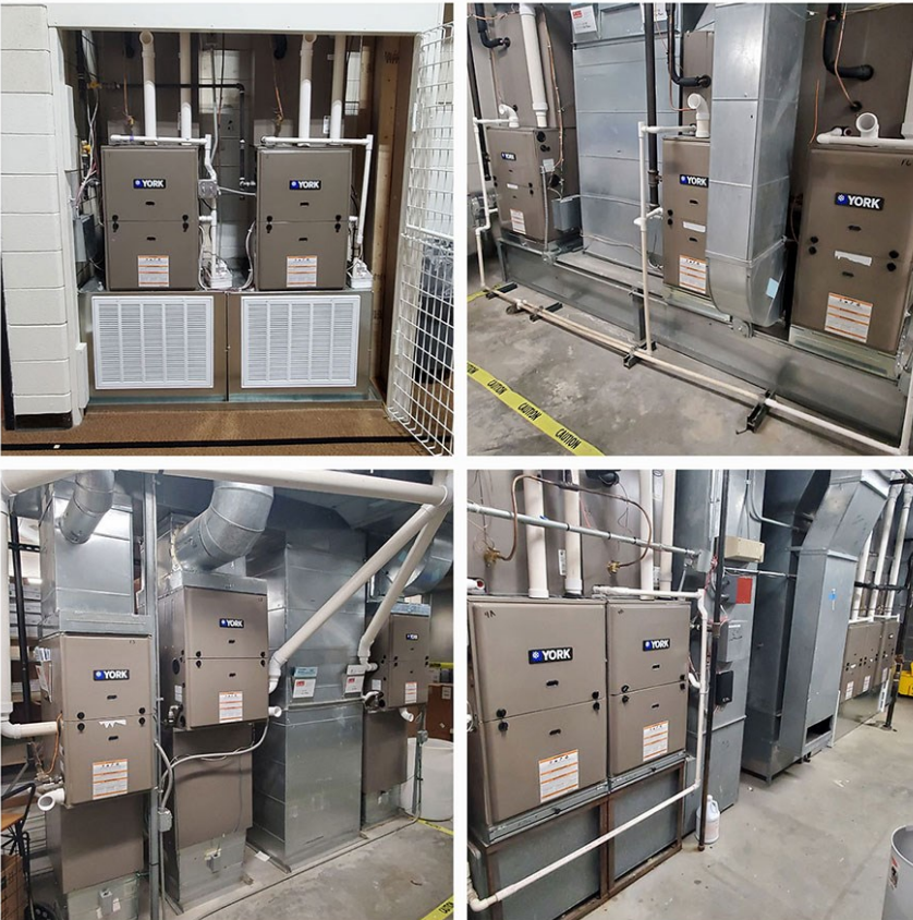
▲ Herren grant dollars were used to assist with the purchase and installation of nine new HVAC systems at Hope Lutheran Church and School in Shawnee.
