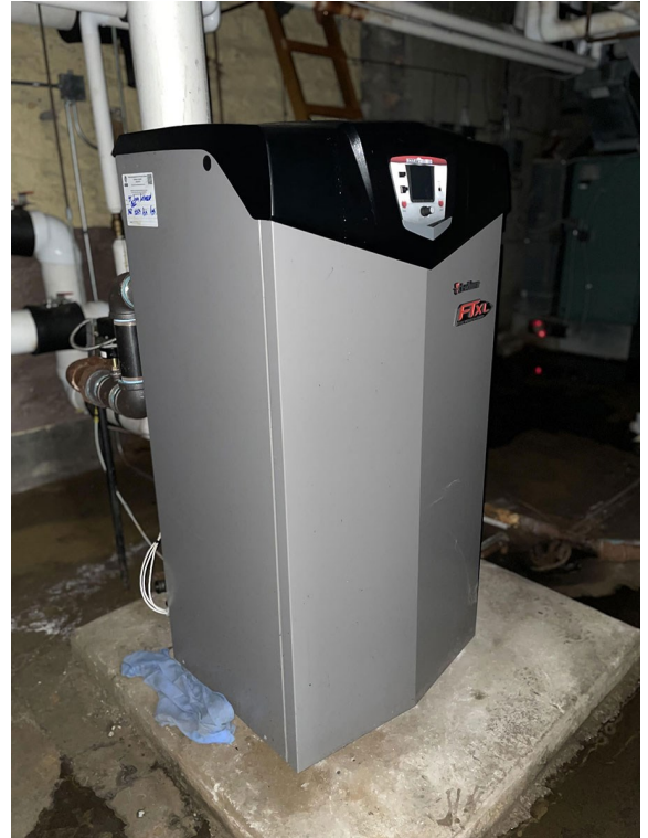
▲ The Herren grant award was used to assist with the purchase and installation of a new boiler at St. John's Ev. Lutheran Church in Topeka.
